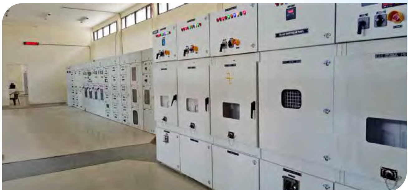
Switch Gear Room
