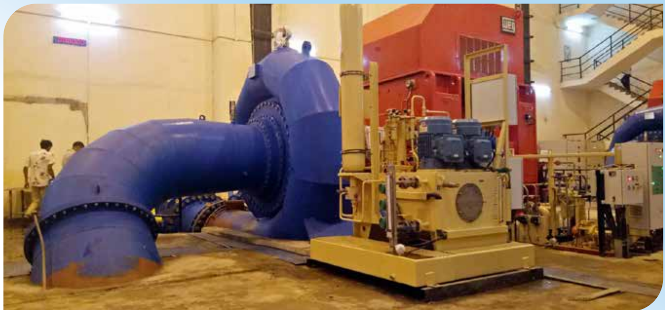
Turbine Generator Unit
